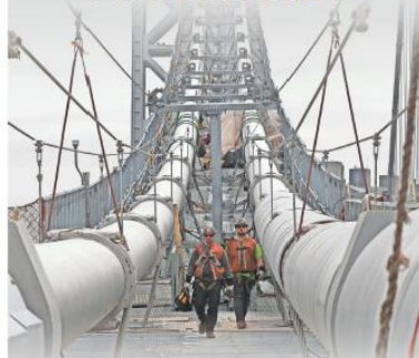
Work crews are reconstructing the "tarrets," the thick cables that hold up the roadway on the bridge that are made up of thousands of thinner wires, some of which are being replaced. The 282 suspended cables are being replaced as well. This is on the north side of the bridge. (USA TODAY NETWORK)
